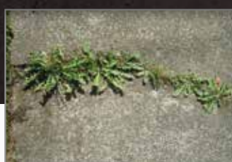
Weeds on pavement
