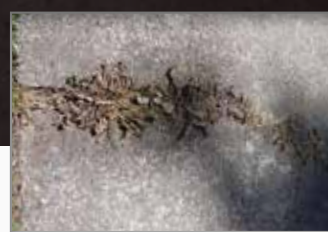
Weeds on pavement 2 - 5 days after treatment
