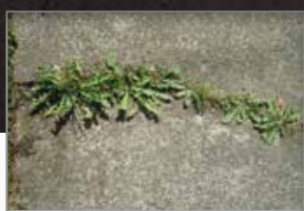
Weeds on pavement
